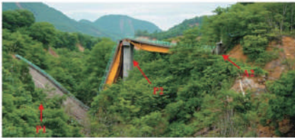
Fig. 3. (a) Sketch of collapsed Matsurube Bridge [22] and (b) in-situ photograph [23].
